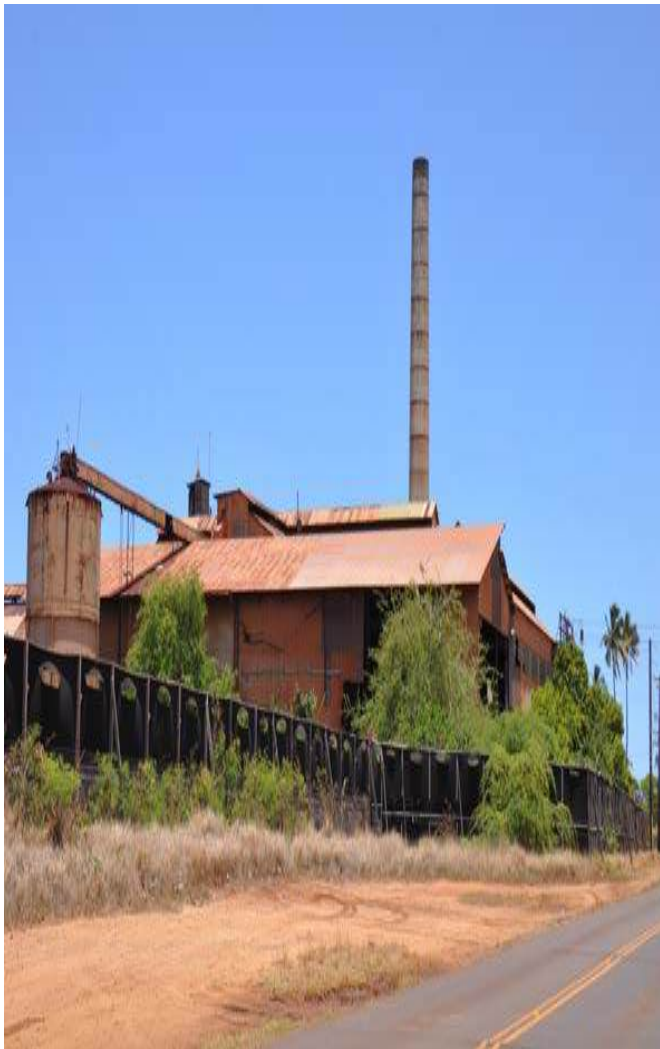
ADC owns thousands of acres across Kauai and Oahu, including former sugarcane lands in Kekaha. (Anita
